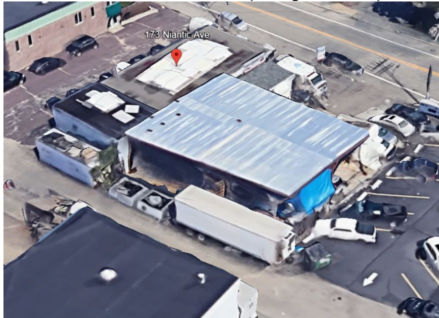
Source: Google Earth accessed on 8/27/2024. Showing storage of materials on roof and in Dewey Avenue.
